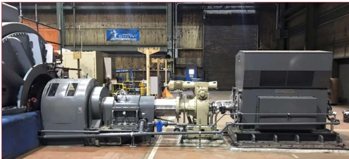
Figure 4.1: Synchronous condenser arrangement with pony motor on right and synchronous machine on left [7]
