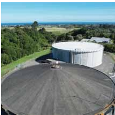
Two drinking water reservoirs, costing $18m, completed at Henwood and Mountain roads to supply Bell Block, Waitara, Lepperton and further north.
