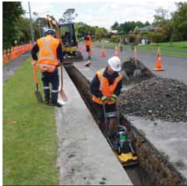
Inglewood's water runs clear again as a $10m project to replace the town's water pipes over three years is completed.
