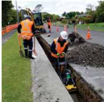
Inglewood's water runs clear again as a $10m project to replace the town's water pipes over three years is completed.
